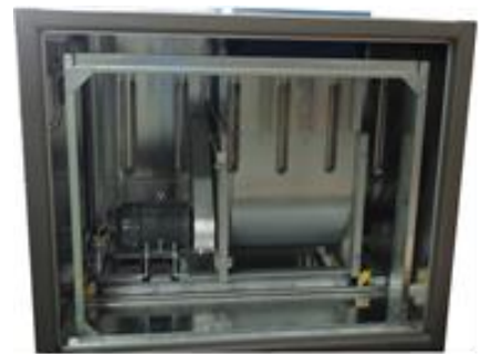
Figure 13. Electric Heater in AHU
